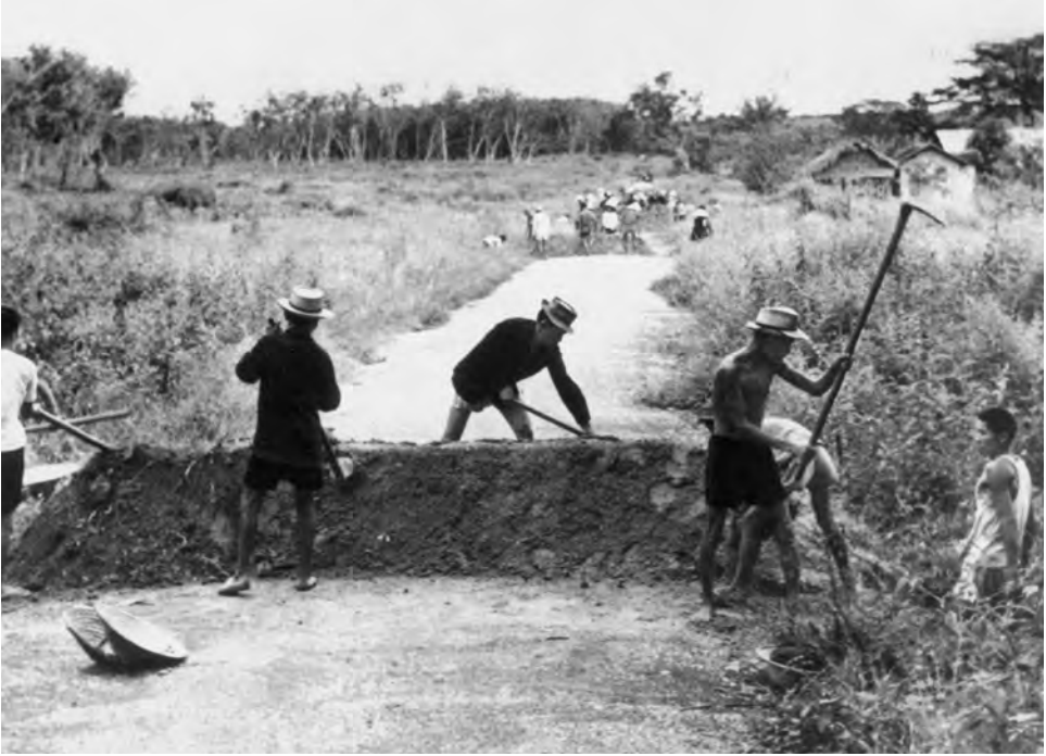
Engineers of the 1st Division encountered obstacles along roads such as the berm under construction by the Viet Cong.
